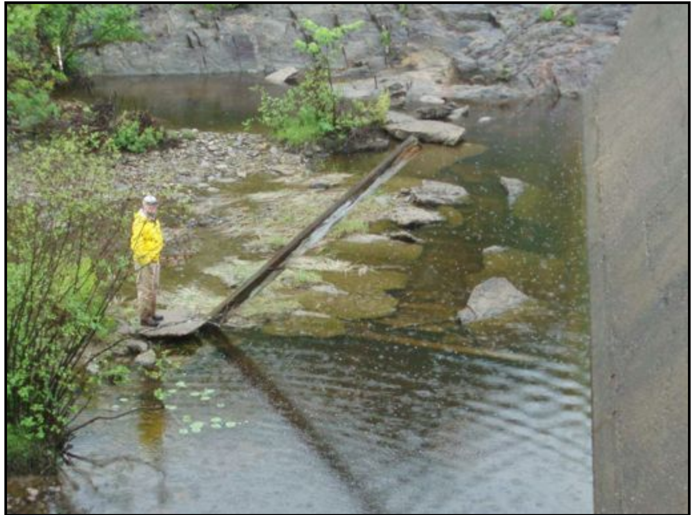
Deteriorated Splash Pad at Base of Dam
